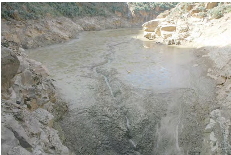
Mud Cake after Gate Blockage during Summer Rains 2007
